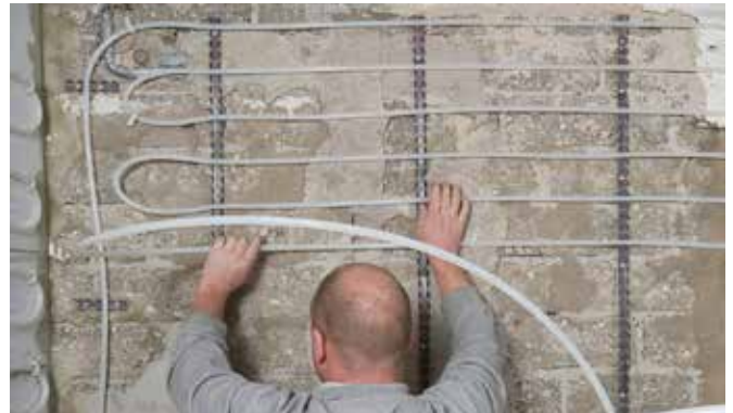
Clicking the heating pipes into the clip rails according to the installation plan
